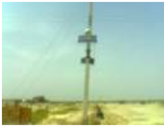
Solar Street Light
